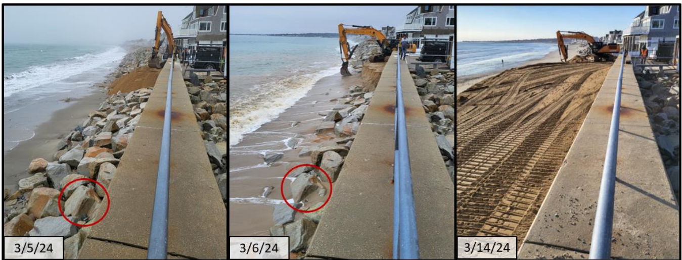
Figure 4: Beach elevation change from before nourishment (left), during the first week of construction (middle), and second week of construction (right). The red circle shows the partial burial of a specific rock in the revetment through natural spreading of the material and the complete burial due to placed nourishment material (source: SCS).
