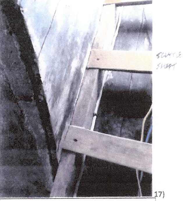
Side view of scuttle with ladder; Dome shaped plastered ceiling of space below the lantern seen on left side.
