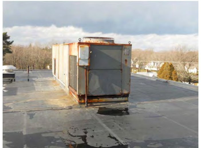
Corroded roof top equipment.
