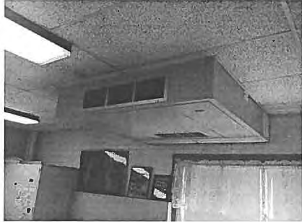
Ceiling-mounted unit ventilator
