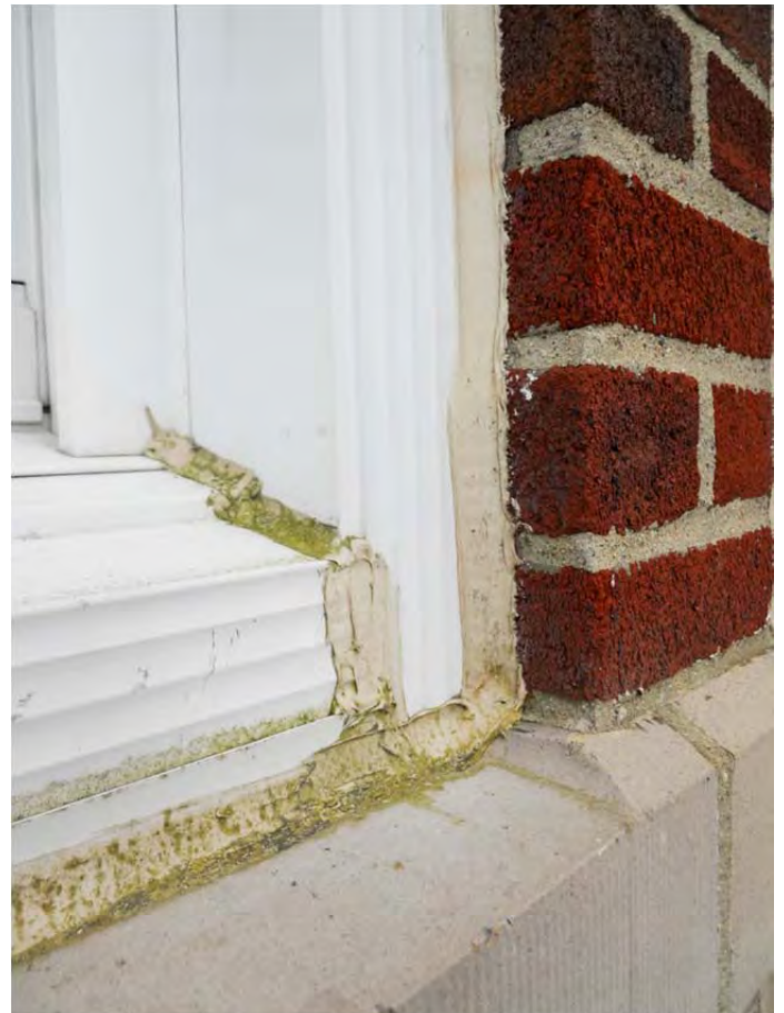
Poor sealant installation and mold accumulation at sealant joints.
