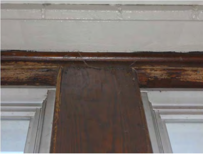
Wood window trim with water damage.
