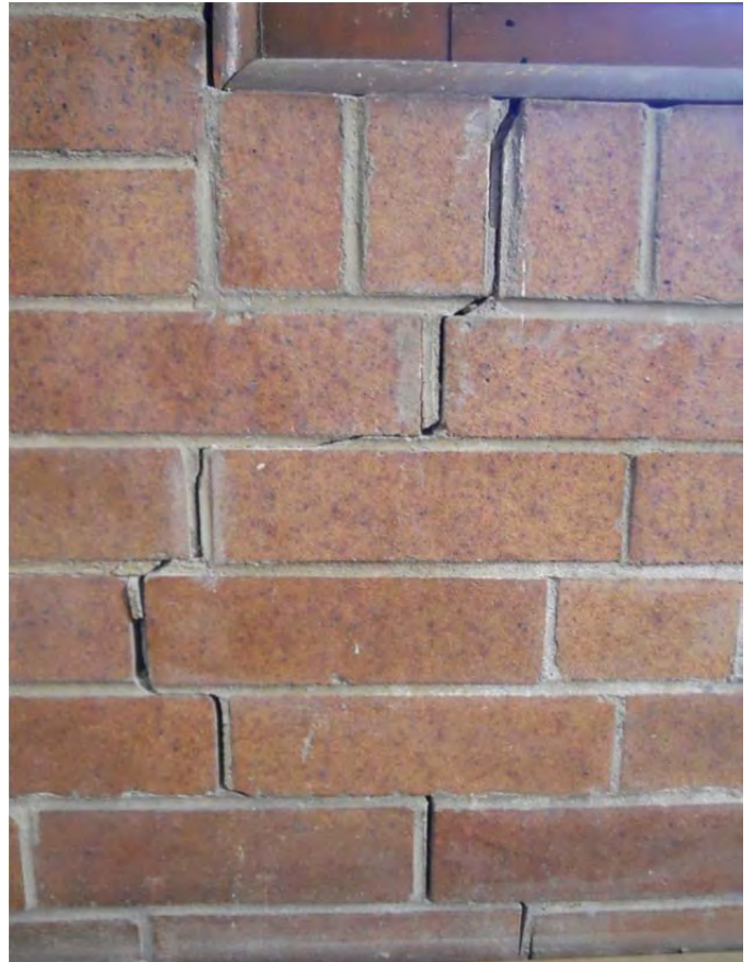
Crack above door head at west elevation in southwest exit stair.
