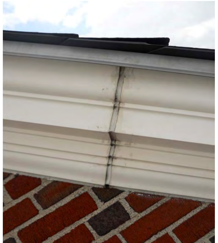
Large sealant joint at butt seam of GFRP raking eave.
