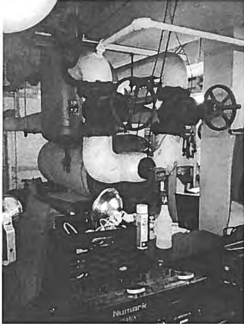
Steam-to-hot water heat exchanger
