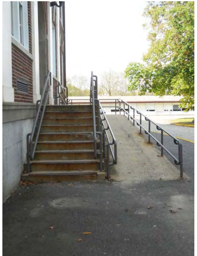
Deteriorated accessibility ramp and stairs at main entry.
