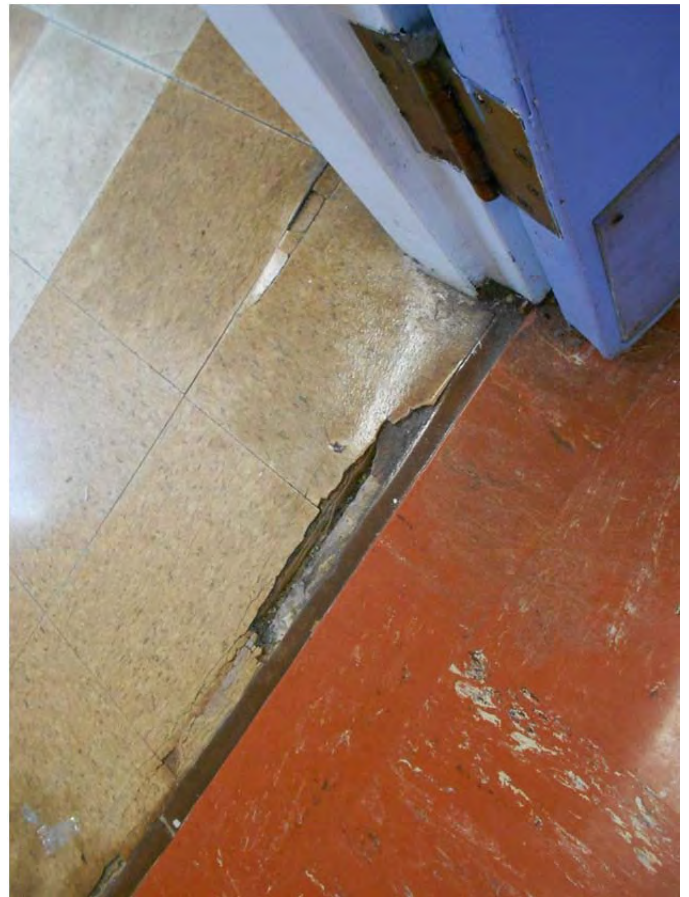
Worn VCT at threshold, evidence of wood beneath VCT.
