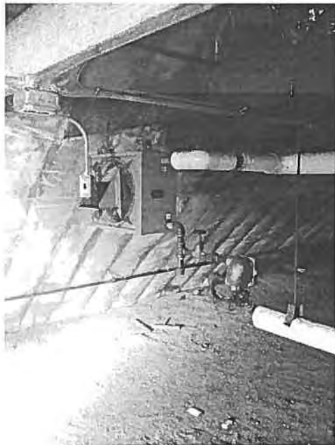
An attic unit heater
