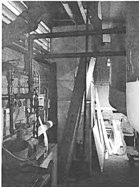
High and low boiler combustion ducts
