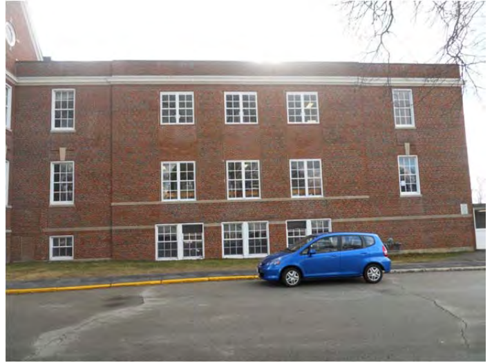
North elevation of west wing with center bay heavily modified where original spandrel windows were removed.
