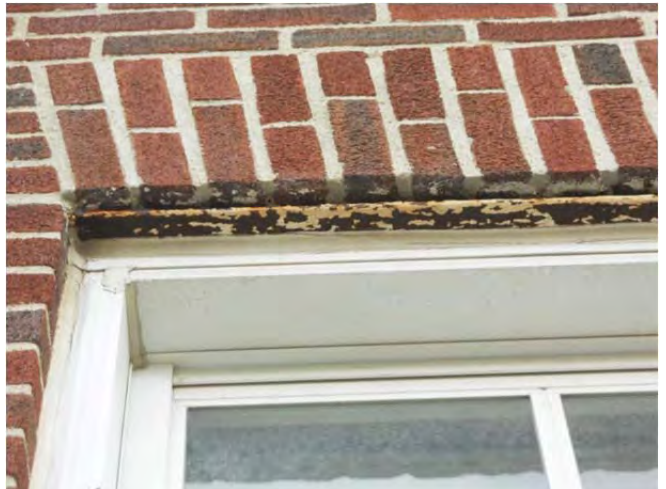
Corroded steel lintel
