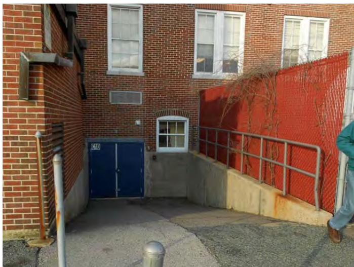
Ramp access outside to the kitchen is extremely steep.
