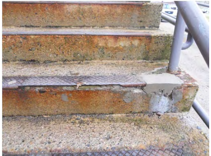
Deteriorated accessibility ramp and stairs at main entry.
