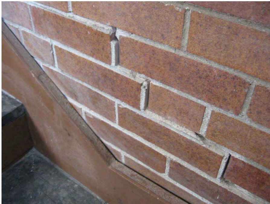
Photo 2.2a – Out of Plane Crack in Southwest Stair Wall
