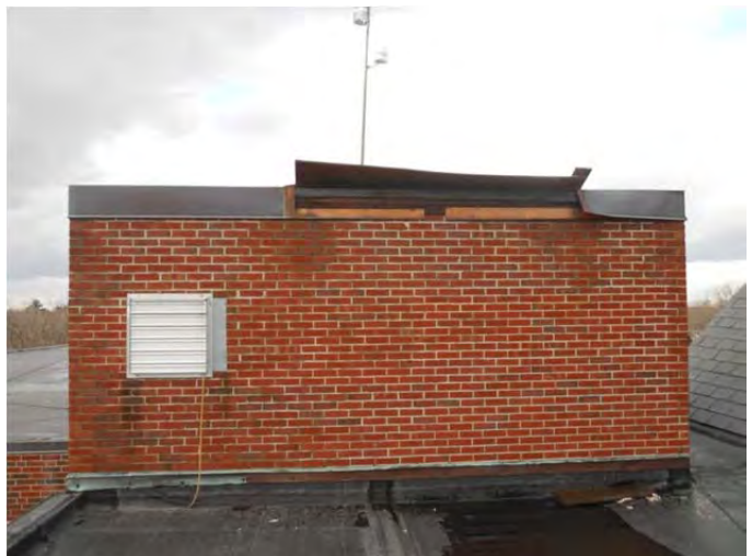
Torn roof flashing at top of elevator.
