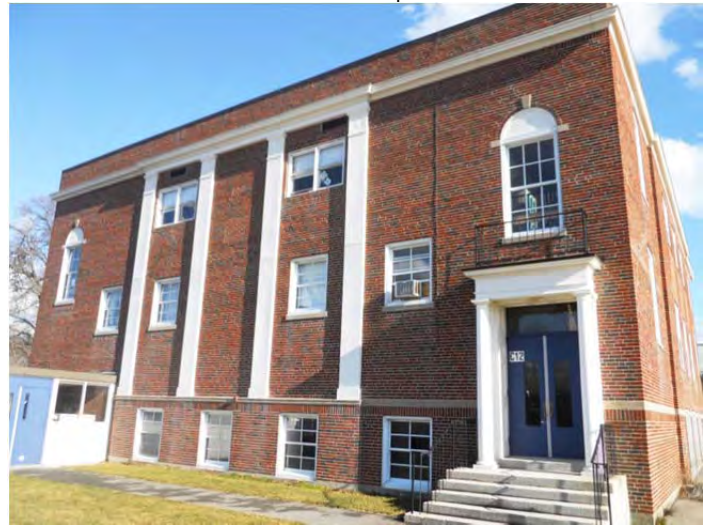
West elevation of west wing heavily modified with non-original window openings.
