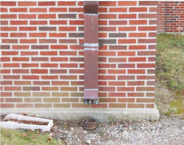
Downspout with no connection to underground system or splash block.
