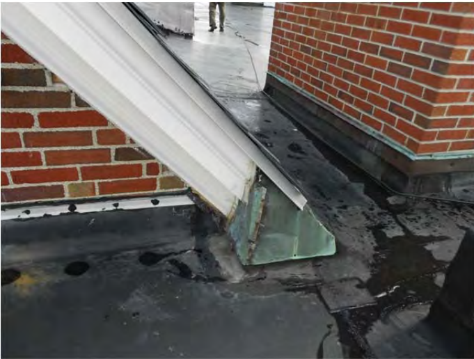
Remaining original copper flashing. Area near elevator over run with wet insulation beneath roof.
