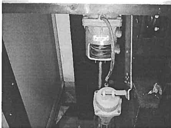
Unit ventilator pneumatic controls (unit interior)
