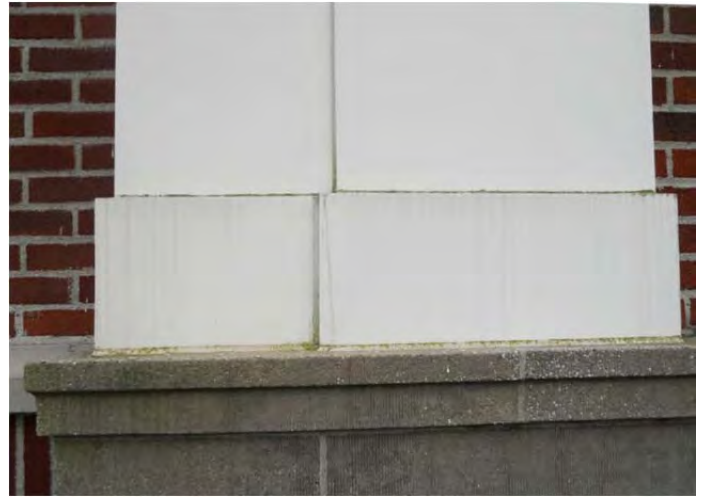
Sealant joints at GFRP with vegetation and mold growth.
