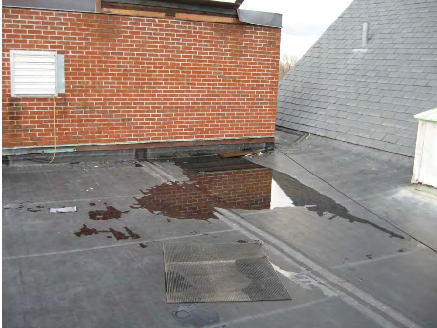
Photo 2.1 – Snow Drifting caused by Sloped Roof and Elevator Mechanical Room
