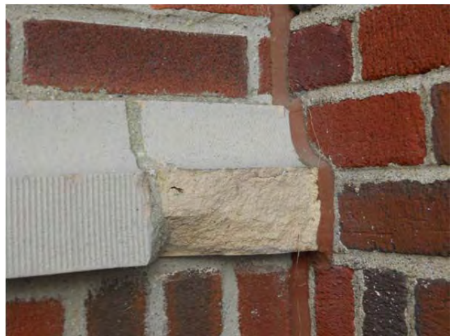
Broken piece of terra cotta
