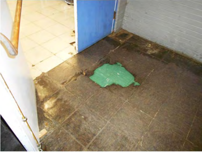
Worn VCT at exit stair, evidence of another layer of VCT beneath.
