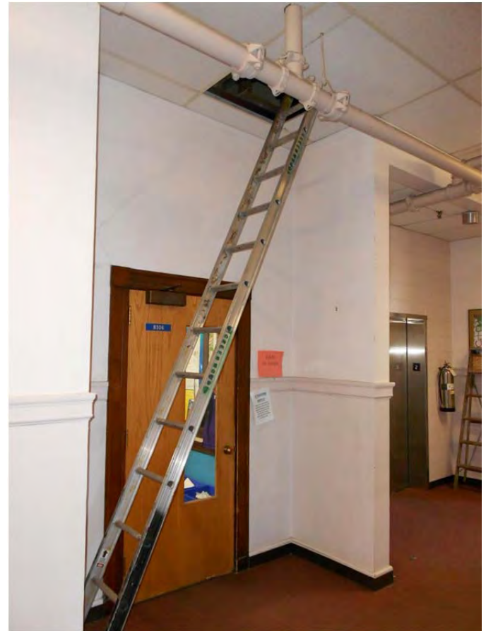
Unsafe attic access.
