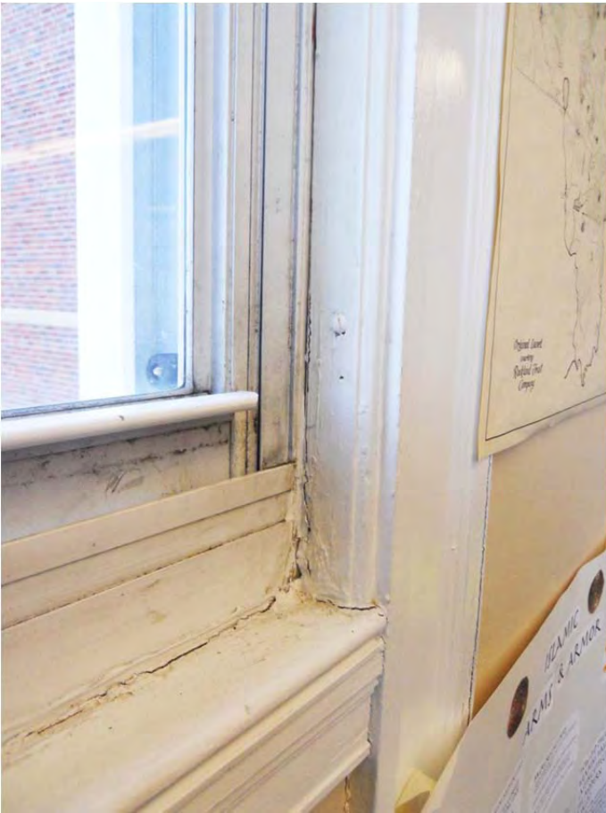
Paint failure at window frame interior.
