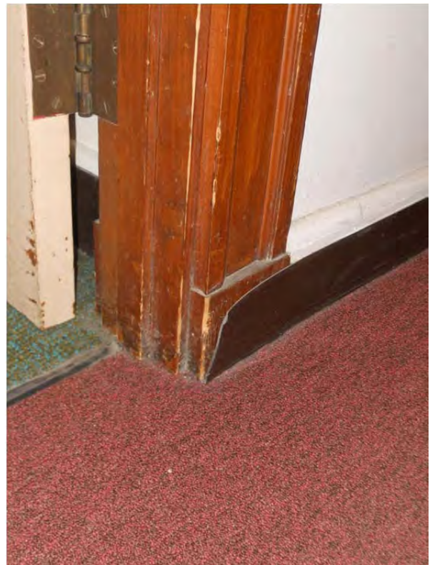
Original door frame and wood base covered with vinyl.
