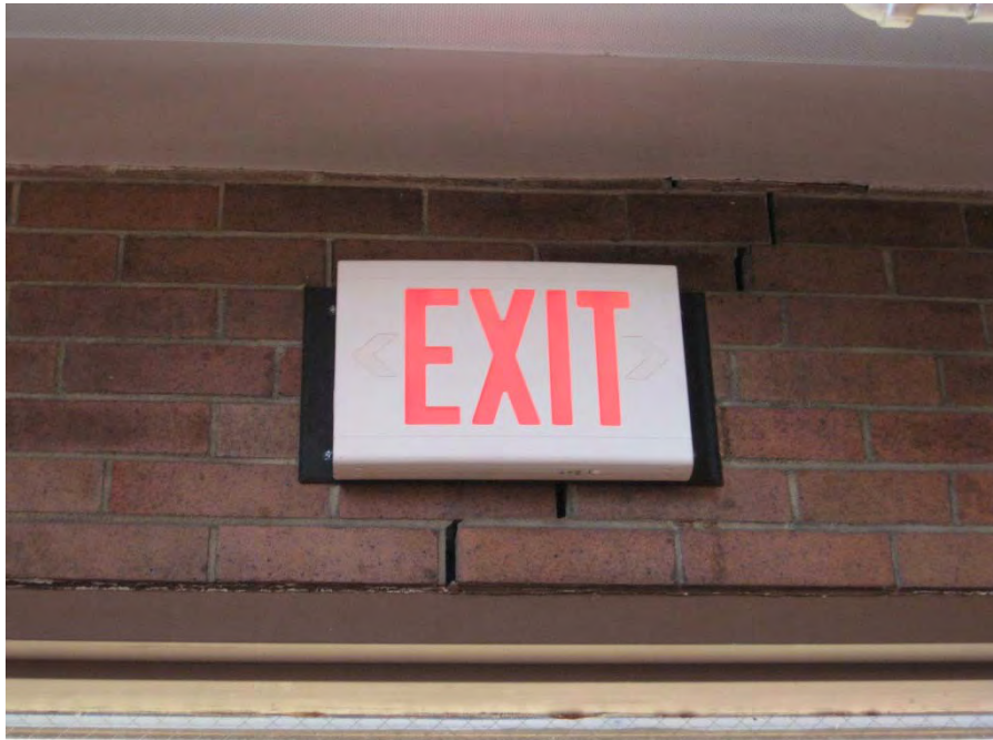
Photo 2.2b – Out of Plane Crack in Southwest Stair Wall
