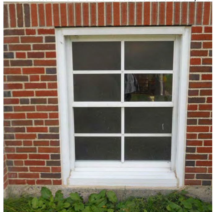
Inappropriate window grid proportions for the style of this building.
