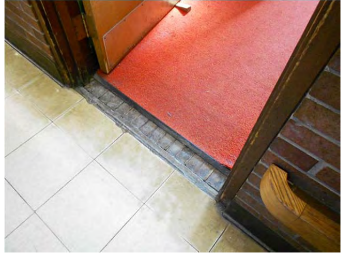
Missing threshold between VCT and carpet, evidence of original wood floor beneath carpet.
