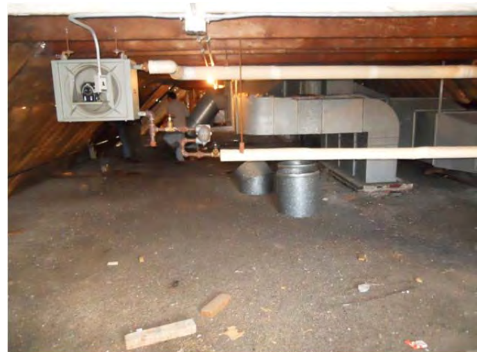
Original tar and gravel roof encapsulated within the attic area. Mechanical equipment existing throughout space.
