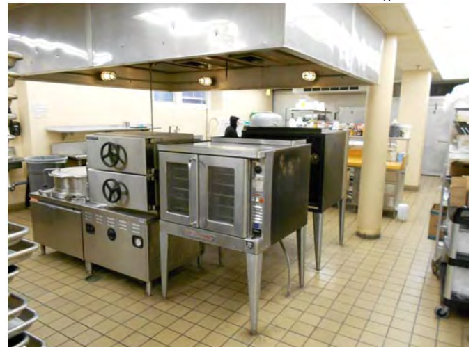
Typical kitchen equipment.
