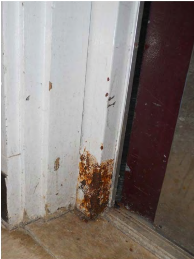
Rusted metal frame, typical condition at all exterior doors.
