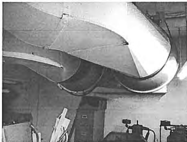
Heat exchanger ventilation system
