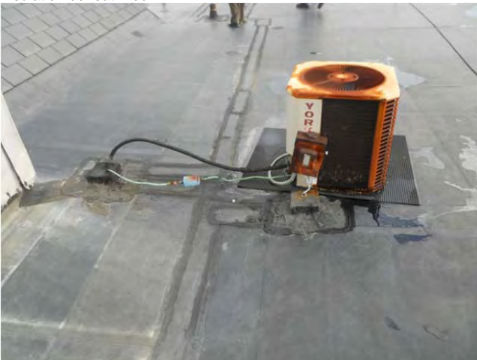
Corroded roof top equipment.
