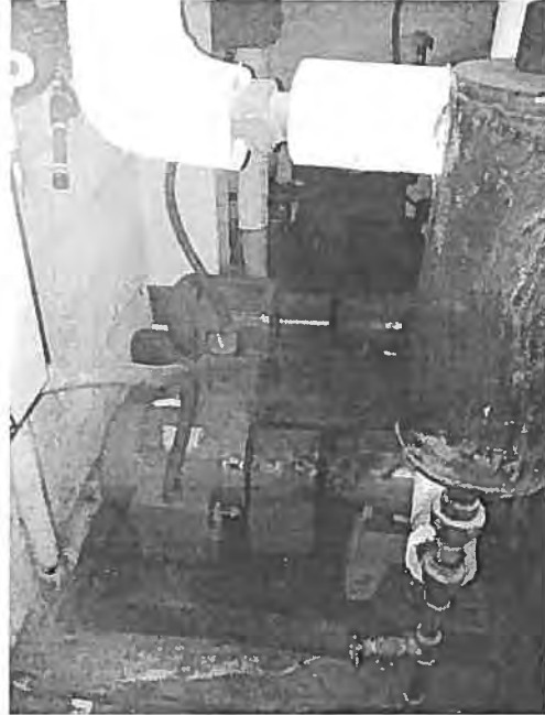
Hot water circulating pumps
