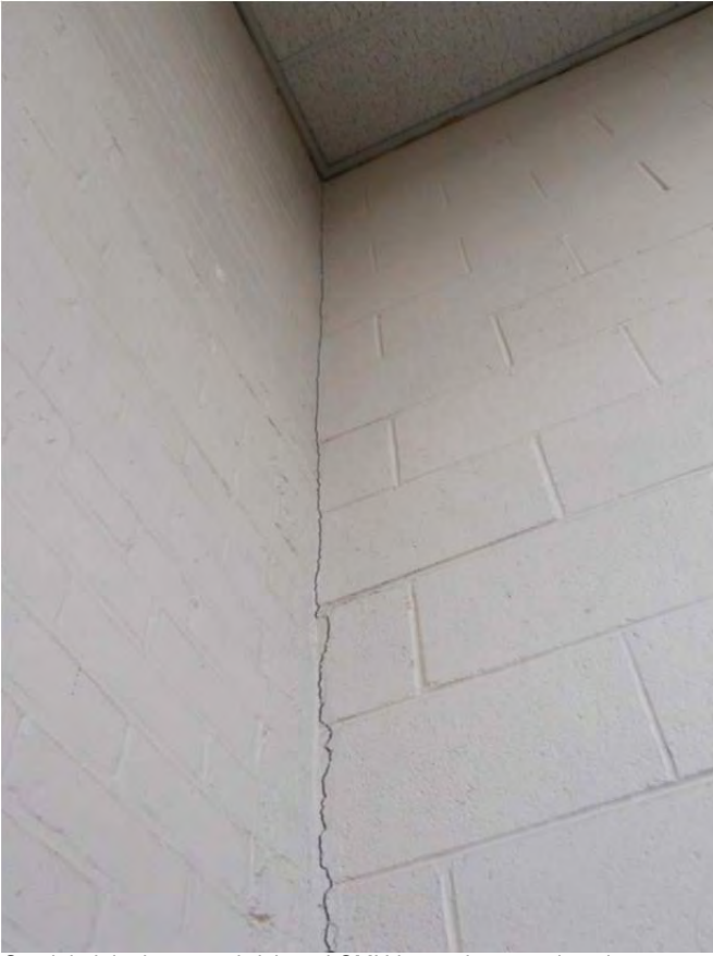
Crack in joint between brick and CMU in southwest exit stair.
