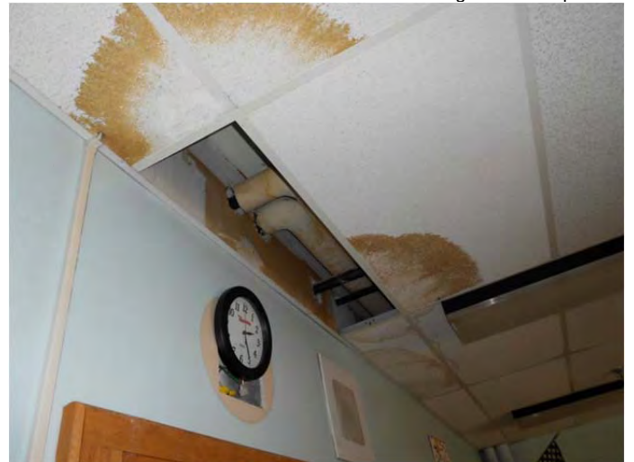
Water leaks visible in ceiling panels.
