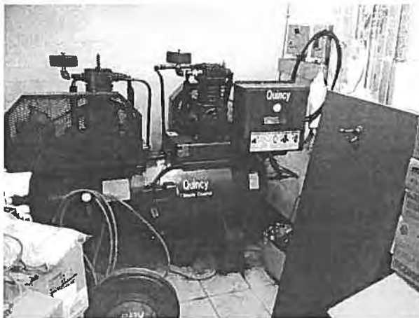
Air Compressor serving school pneumatic controls
