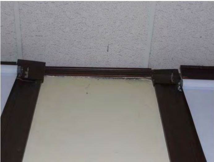
Wood window trim with water damage.
