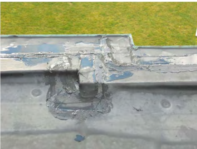
Coping at flat roof with EPDM seam on top of metal coping and demonstrating much past maintenance.
