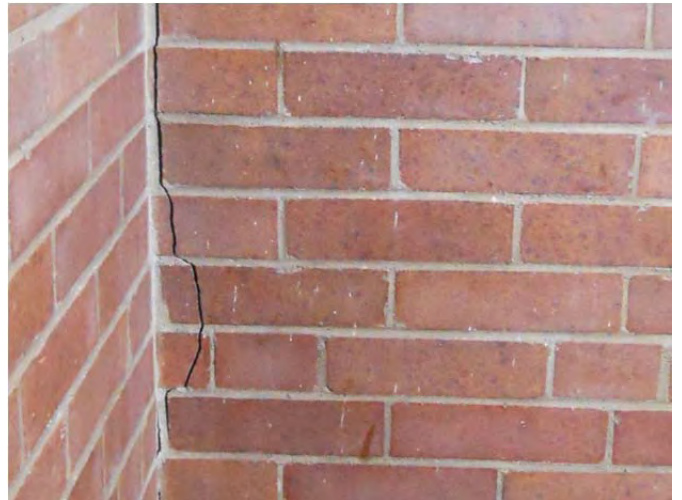
Crack in brick wall at southeast corner of southwest stair.
