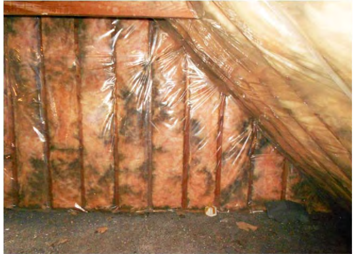
Attic insulation covered in mold.
