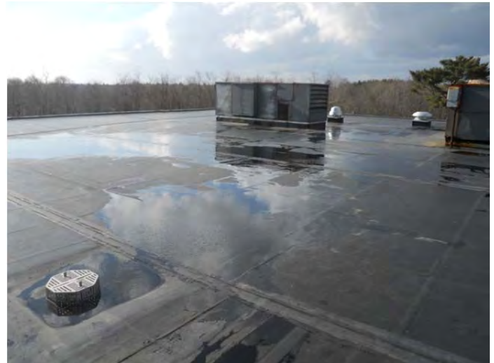
Ponding of water at EPDM roof at west wing.
