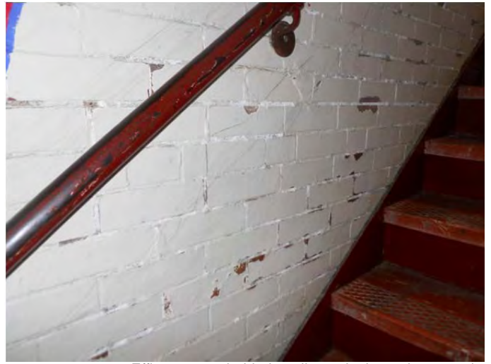
Efflorescence behind peeling paint in northwest stair.
