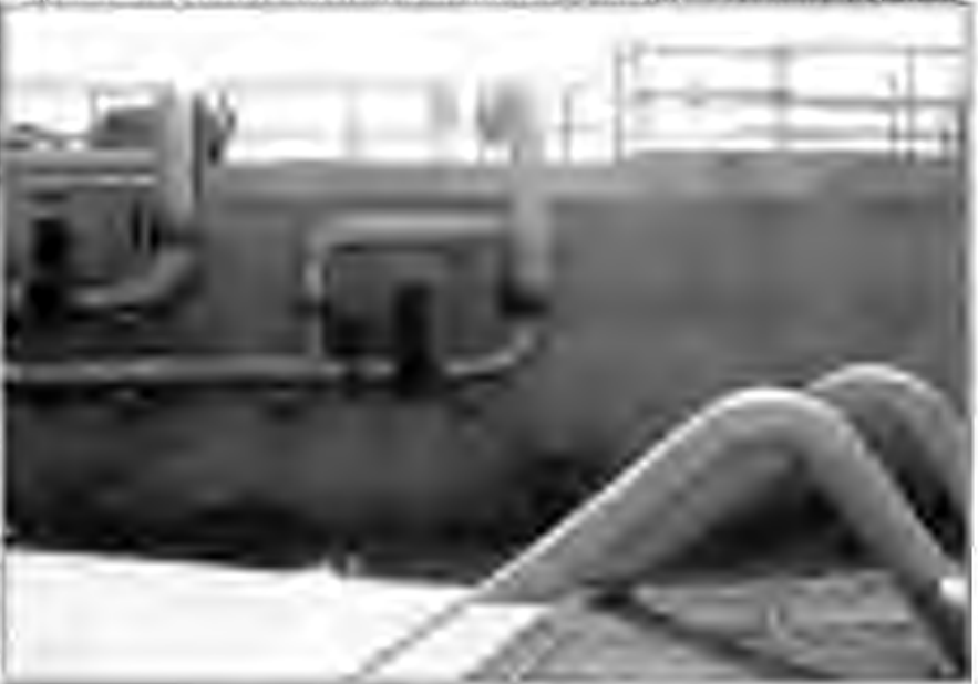
Figure 4 – Island Road Wastewater Treatment Plant (UK) – Eccentric Plug Valves
