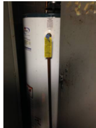
Domestic Water Heater
