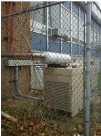
Generator at Town Hall
