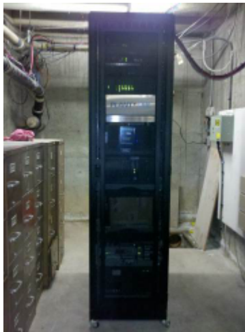
Emergency Communications Rack
