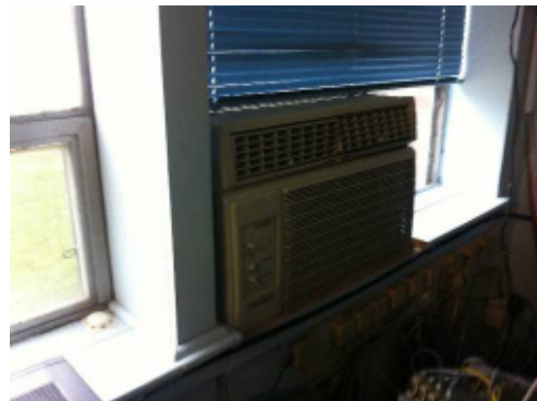
Window AC Unit
