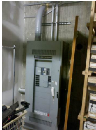
Main Distribution Panel
