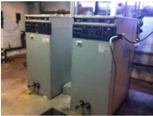
Gas Fired Boilers
