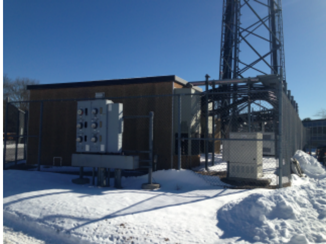
Figure 3: Cell tower and electrical and generator equipment north of the Police station
