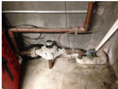
Domestic Water Service & Meter
