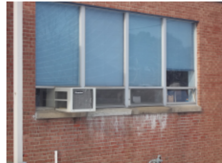
Efflorescence at Window Sills
