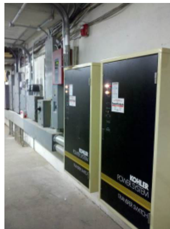
Transfer Switches at Town Hall
