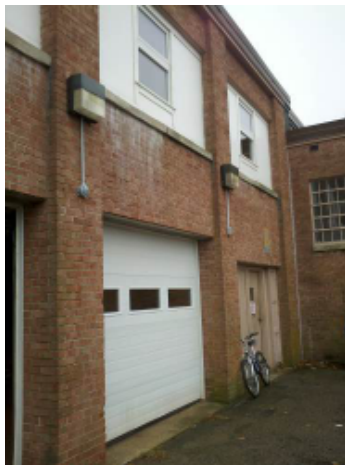
Building Wall Packs
