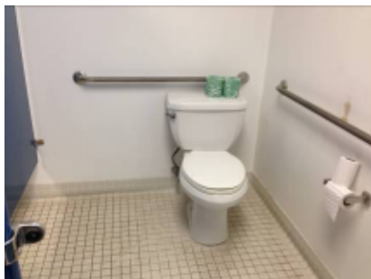
Floor Mounted Water Closet
