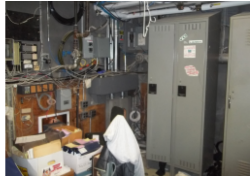
Personnel Lockers in Electrical Room
