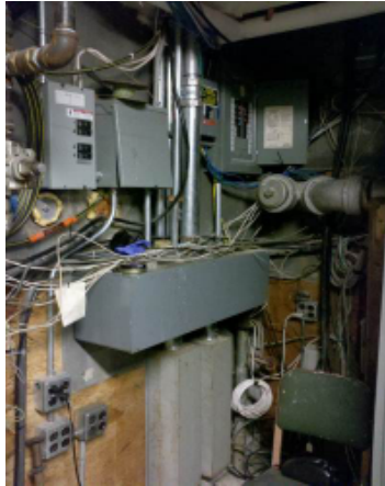
Electrical Panels & Sewer Lines
