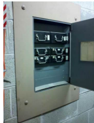
Original Fusible Panel
