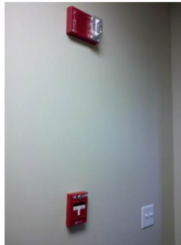
Horn/Strobe & Pull Station
