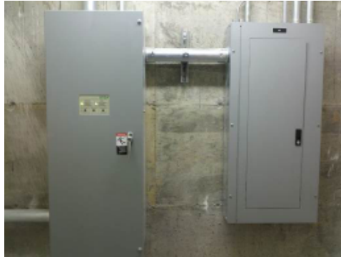
Automatic Transfer Switch & Panel
