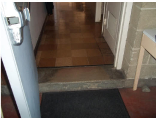
Step between App Bays and Living Quarters
