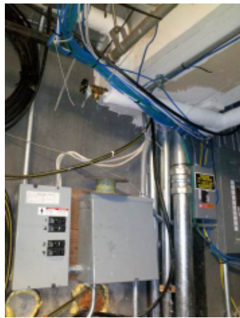
Tel/Data Wiring Bundle
