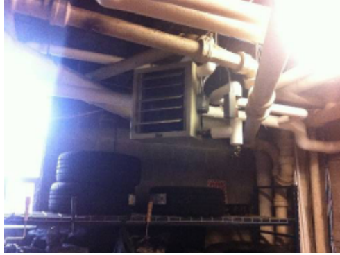
Hot Water Unit Heater
