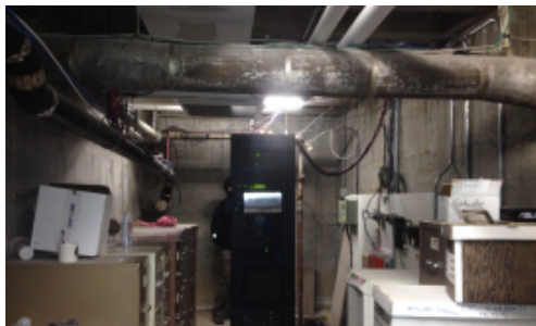
911 Telecomm Rack in non-ventilated Storage Room
