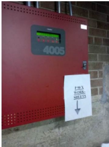
Fire Alarm Panel
