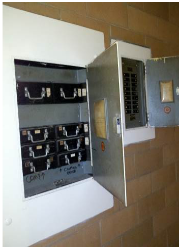
Flush Main Panel
