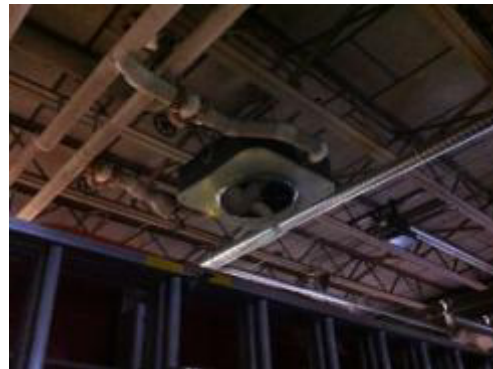
Ceiling Unit Heaters
