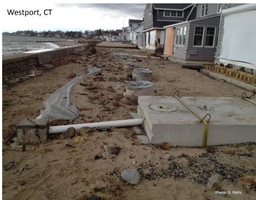
Figure 22 Exposed septic system after coastal storm, CT.
