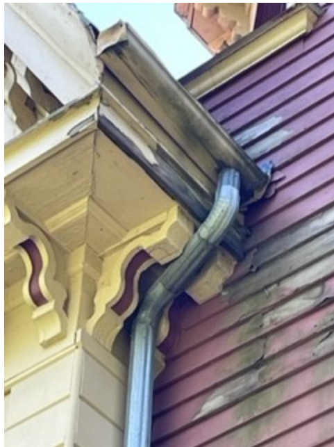
Ellis tower, Gutter, overflow problems
