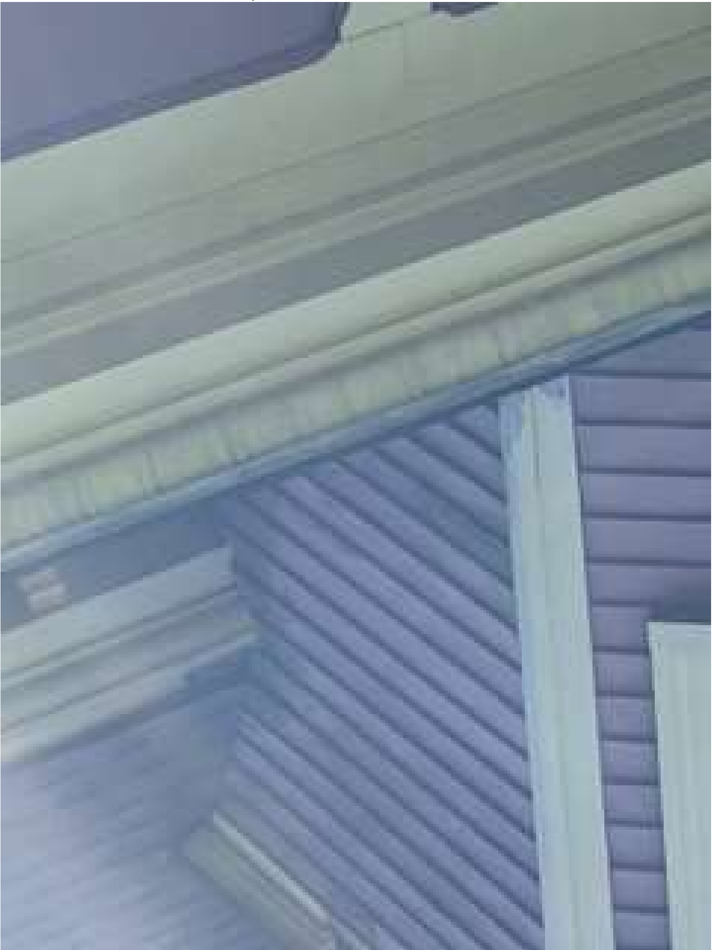
Ellis tower, water control issue other side
