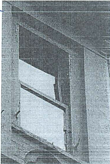
49. Northeast fac;;ade - Tower detail: Deteriorated wood trim
