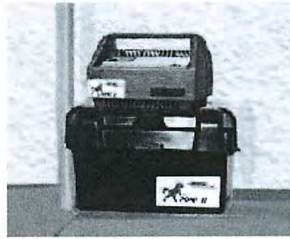
Minimum 8 hour battery back-up units
