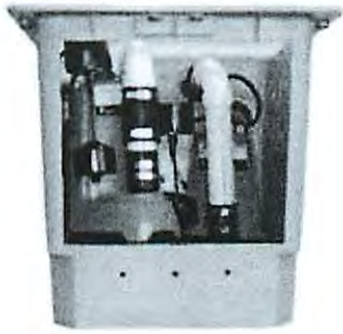
Perforated Sump, pump and backup pump
