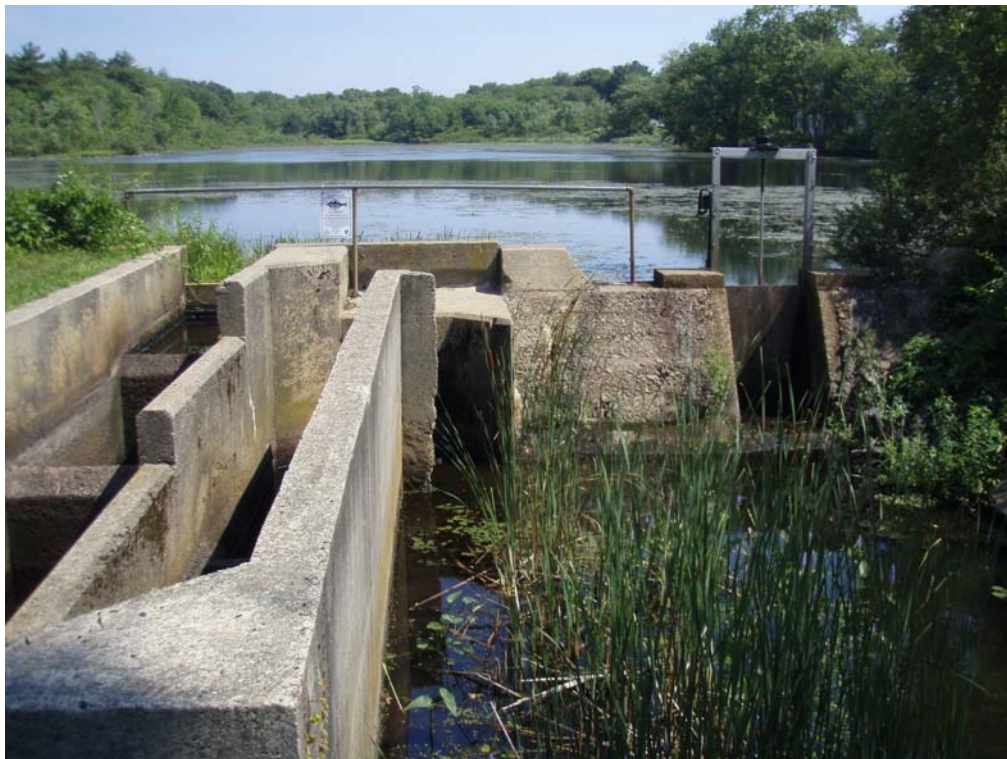
Figure 4. Fish ladder and low level outlet structure at Old Oaken Bucket Pond.
