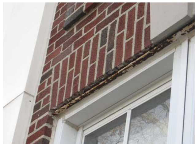
Deteriorating lintel at B-Wing.
