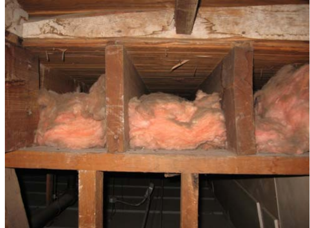
Wood joists supported on wood studs -typical floor framing at B-Wing (1917 Building).
