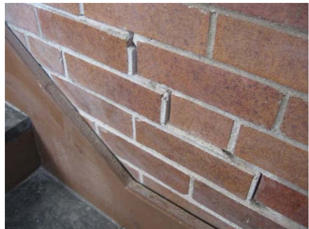
Out of plane cracks adjacent to southwest stair (B-Wing).
