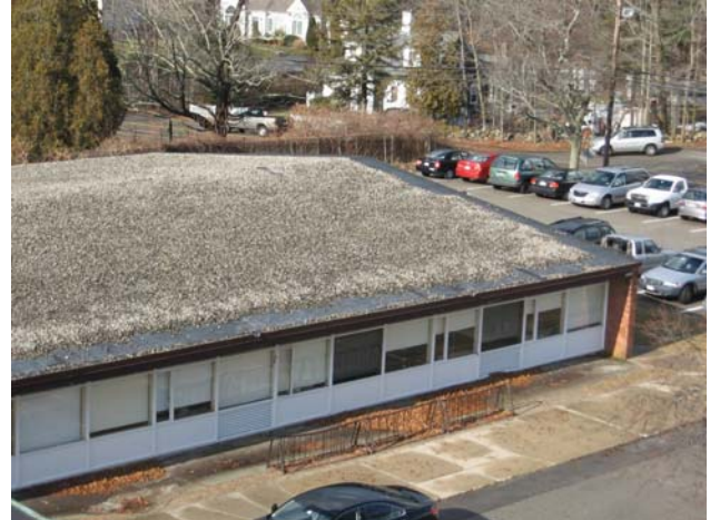
Missing roof ballast along roof edges (C-Wing).
