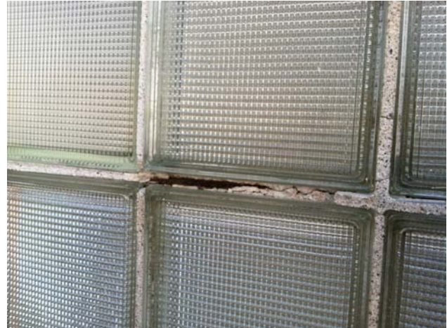
Rusting steel supports in glass block mortar joints at upper gymnasium wall (A-Wing)
