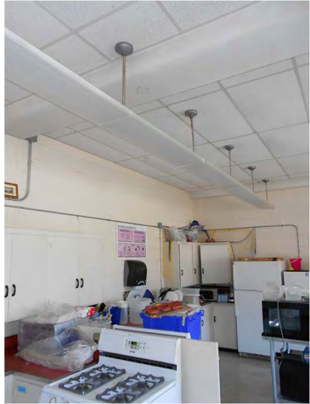
No ventilation hoods over cooking appliances
