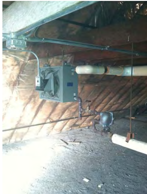
An attic unit heater
