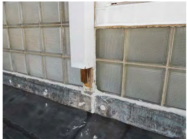
Extensive sealant & missing pilaster at gym
