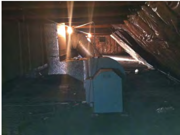
An exhaust fan located in the attic of the original building
