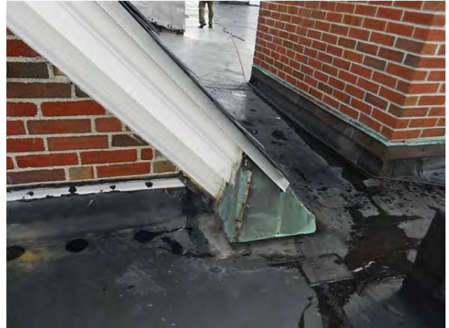
Remaining original copper flashing at area near elevator where spongy insulation was noted
