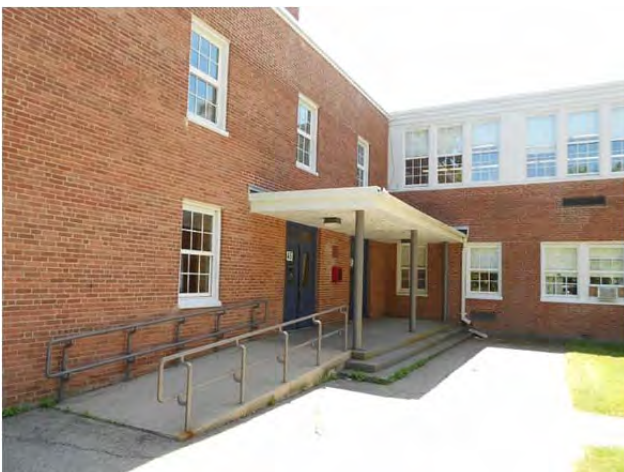
Gymnasium lobby entrance is generally Code compliant except for handrails at the stairs.
