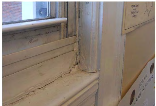
Paint failure at window frame interior in B wing
