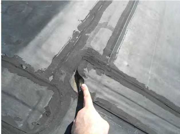
Extensive sealant & missing pilaster at gym
