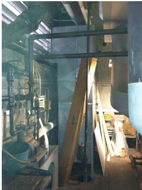
High and low boiler combustion ducts
