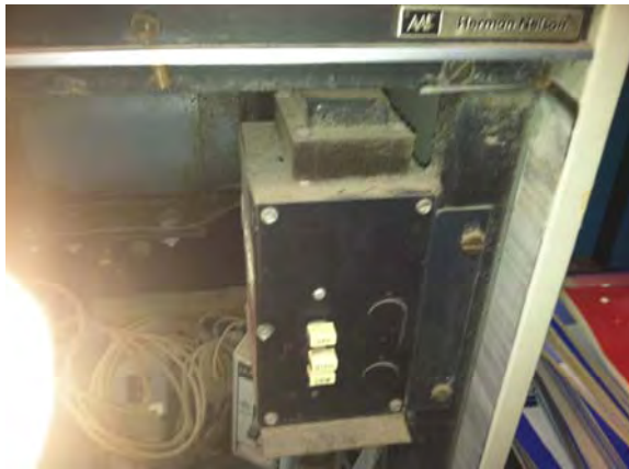
Interior of an AAF Herman Nelson unit ventilator
