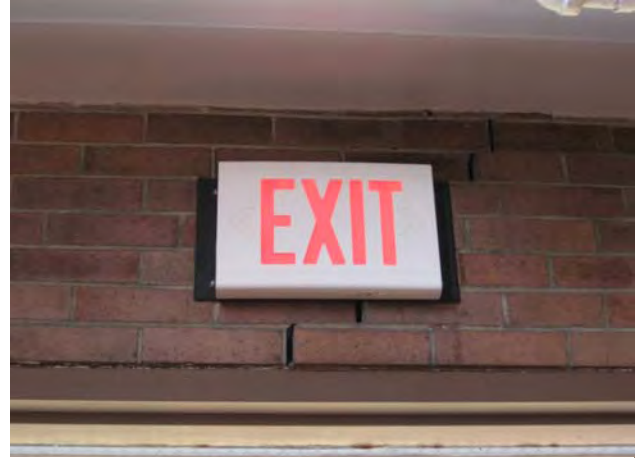
In-plane cracks over door in southwest stair (B-Wing).
