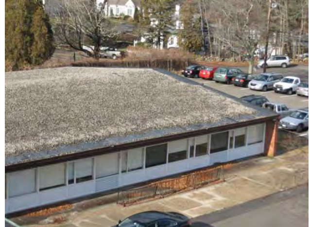
Missing roof ballast along roof edges (C-Wing).
