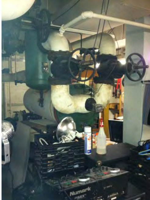
Steam-to-hot water heat exchanger
