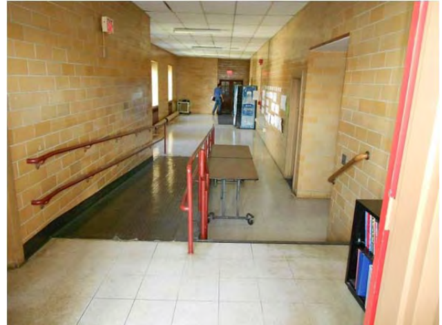
The upper gymnasium lobby ramp appears to be a more recent renovation and is generally compliant
