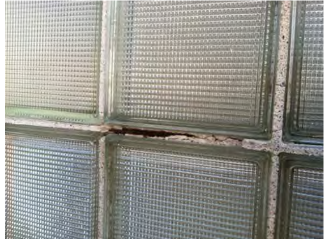
Rusting steel supports in glass block mortar joints at upper gymnasium wall (A-Wing)
