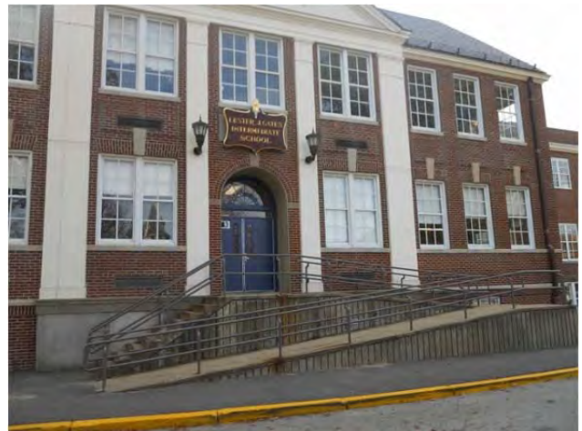
Main entrance stair and ramp at B wing has significant compliance issues.
