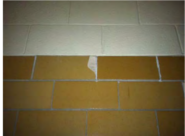
Random spalling of interior face of glazed block.
