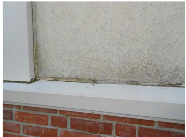
Sealant joints at the stucco are dirty and failing
