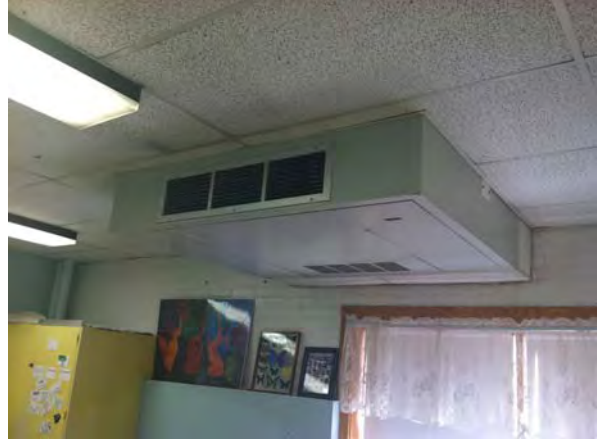
Ceiling-mounted unit ventilator
