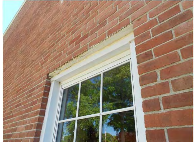
Lintels in A wing are rusting and require prep and repaint before deterioration accelerates
