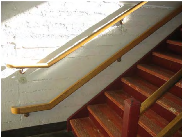
Some wall-mounted handrails are compliant, albeit sporadic. The lower rail is not required nor compliant.
