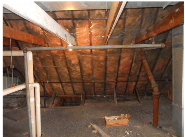
Access to the attic in B wing is located at in the eave space, limiting ease of access.
