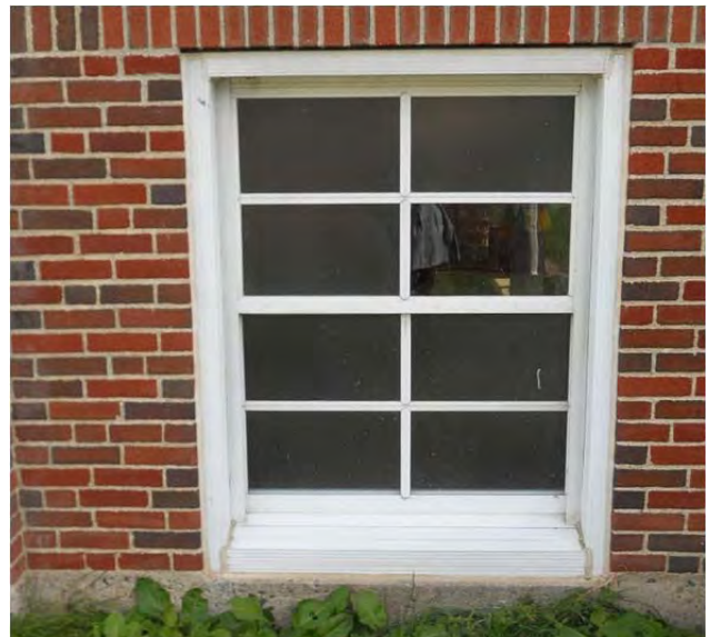
Inappropriate window grid proportions for the style of this building
