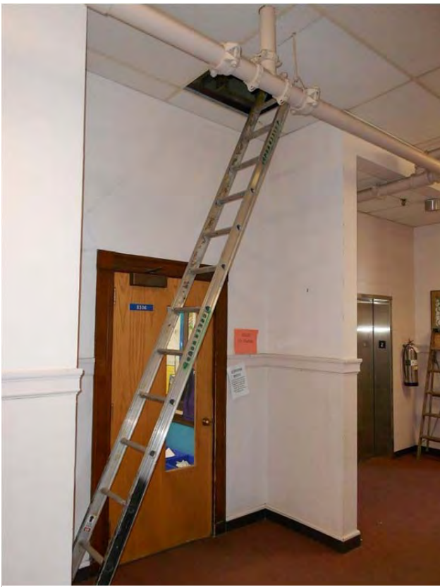
Ladder access to B wing's attic is dangerous for both workers and building occupants.
