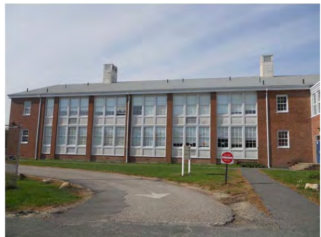
Original wood "curtainwall" covered with aluminum panning. Solid panels are coated with stucco.
