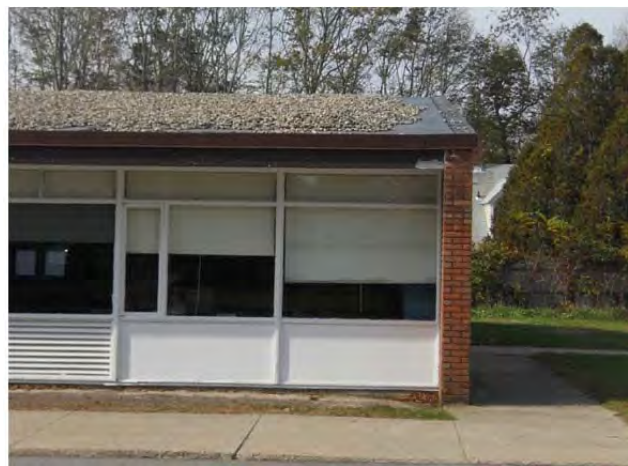
C wing roof showing missing ballast at roof edges
