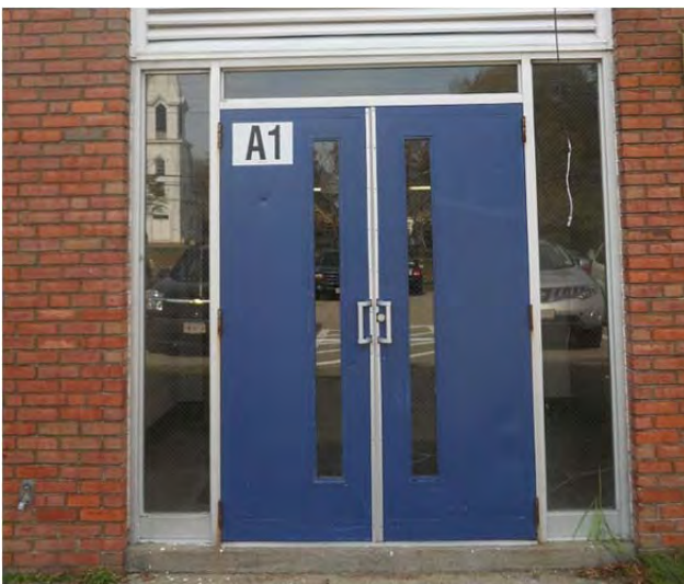
Antiquated hardware and plate glass mean the doors should be replaced
