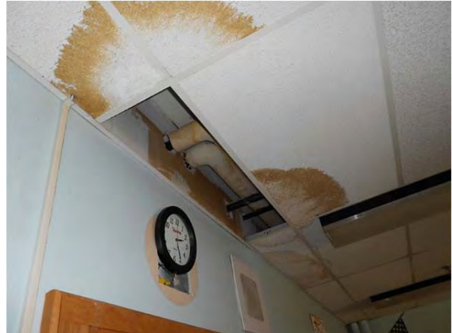
Existing ceilings throughout the building are stained from roof and steam pipe leaks.
