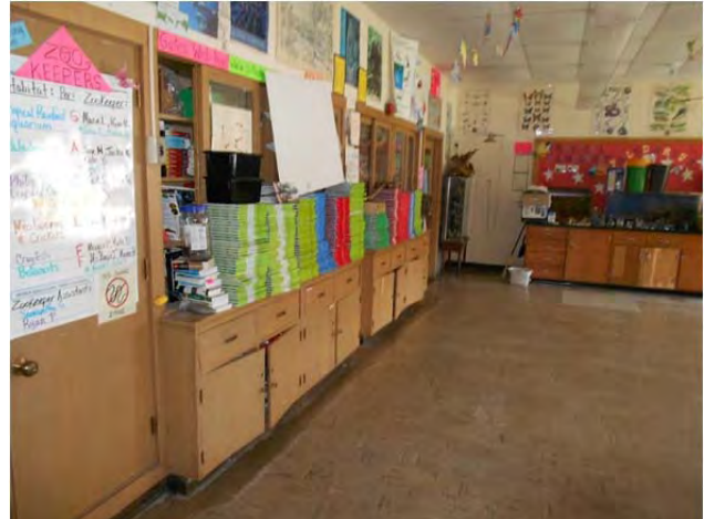
A wing casework is still serviceable but is nearing the end of its useful life
