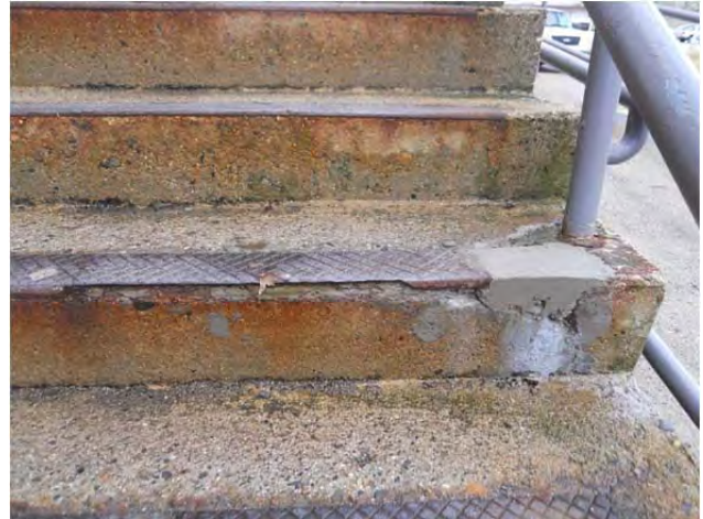
Main entrance stairs and ramp at B wing have rust jack and patch failures.
