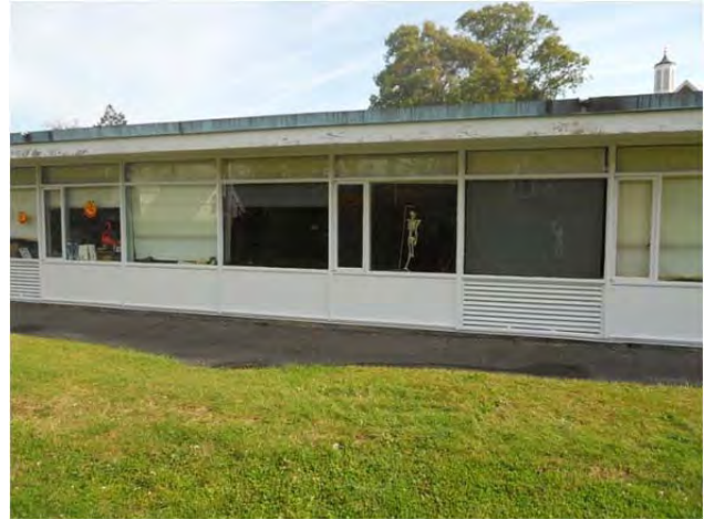
C wing roof edge is bent and failing in many locations
