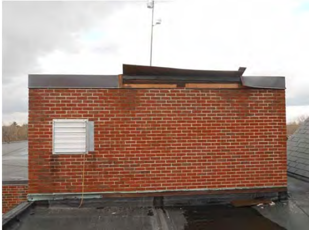
Torn roof flashing at the top of the elevator shaft
