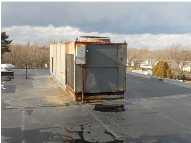
Corroded rooftop equipment dating back to the 1974 renovation
