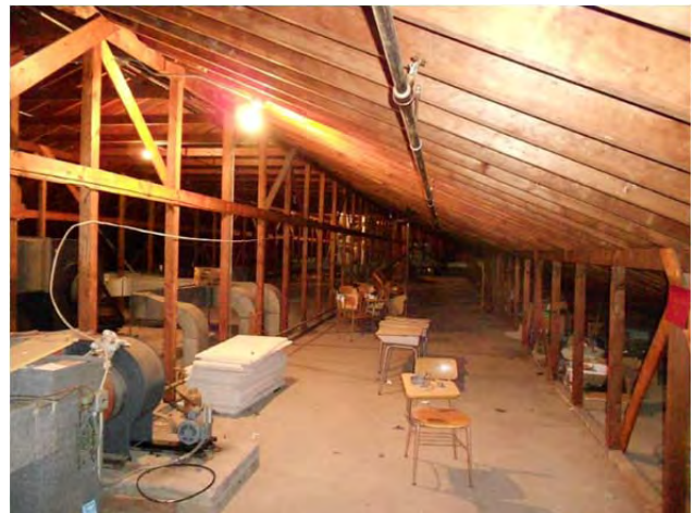
Even the eave space in A wing's attic has plenty of height.
