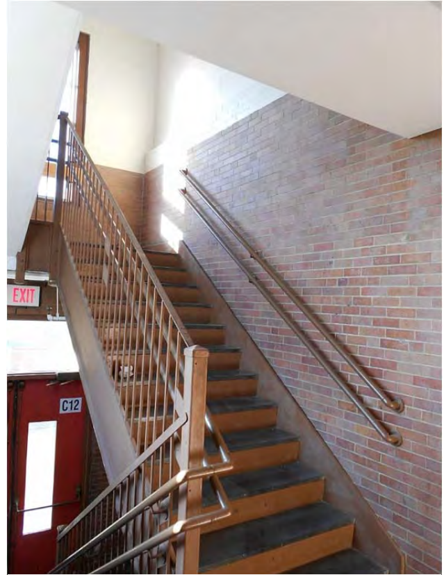
Some stairs are closer to compliance than others. Still, the handrails do not have the proper extensions.
