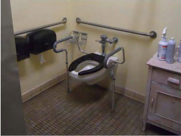
Handicapped compliance has been attempted to be met in non-compliant ways
