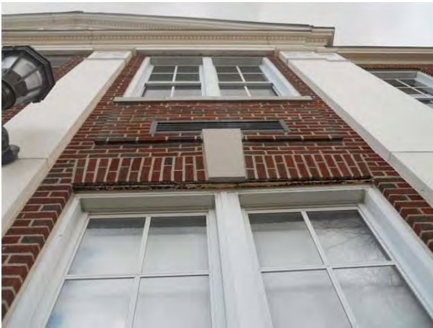
Main entry elements fabricated of GFRP such as pilasters and pediment
