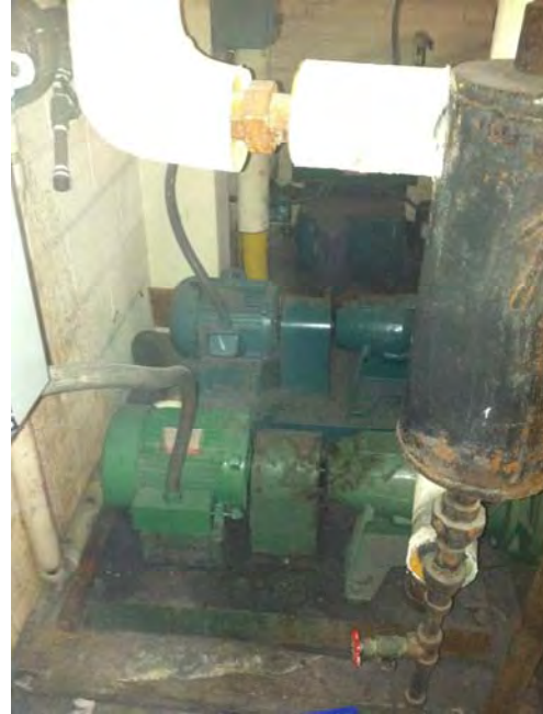
Hot water circulating pumps
