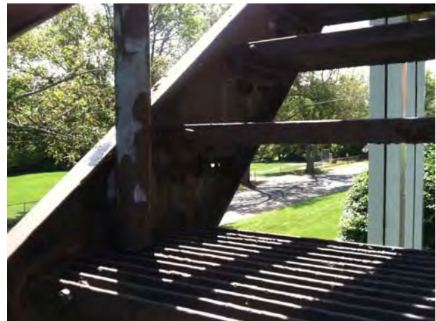
Deteriorated steel stringers and treads at gymnasium east egress exterior stairs.
