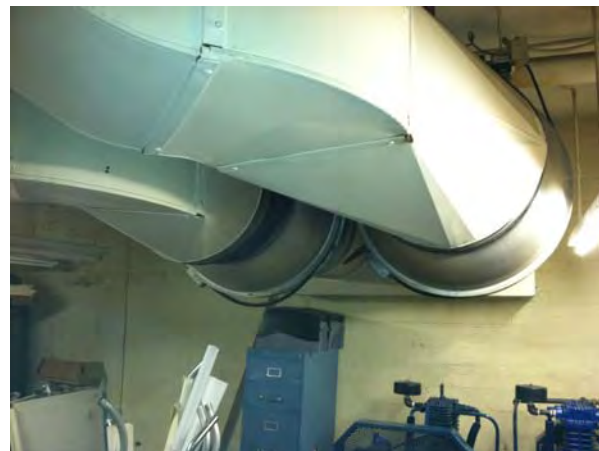
Heat exchanger ventilation system
