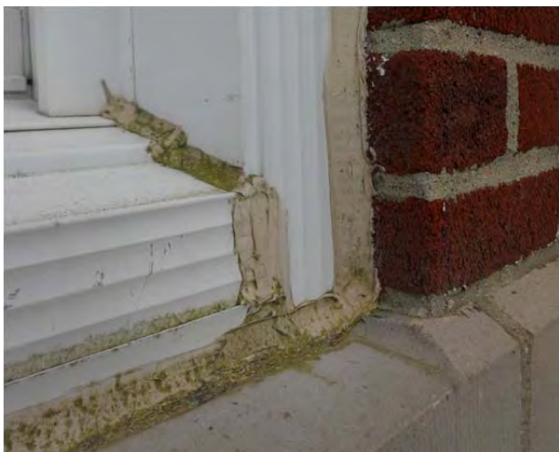
Poor sealant installation, mold accumulation, and staining at sealant joints
