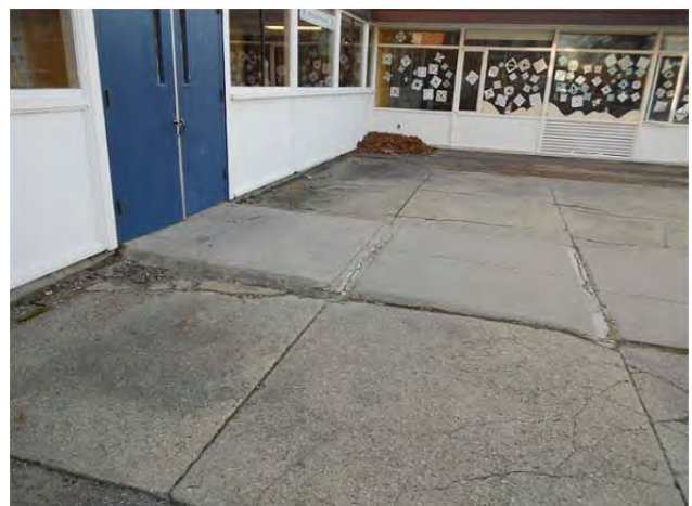
Although handicapped compliant, the sloped walk is cracked and heaved in several locations.
