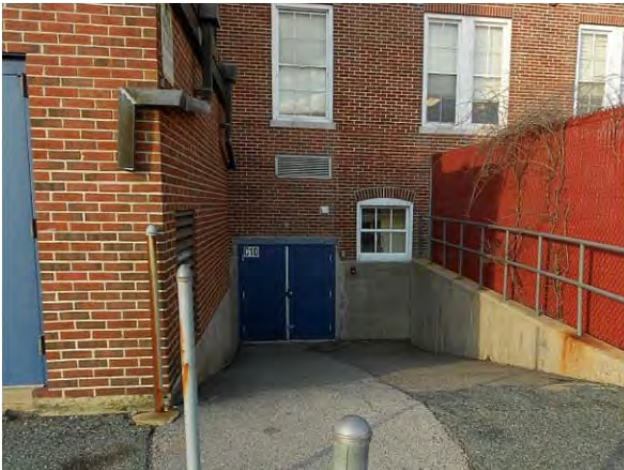
The kitchen loading door has an extreme pitch outside that promotes water infiltration
