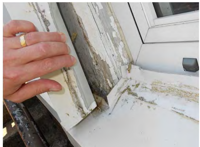
Loose panning around original trim at A wing can compromise existing substrate(s)
