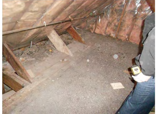
The original tar and gravel roof remains in place in the B wing attic.
