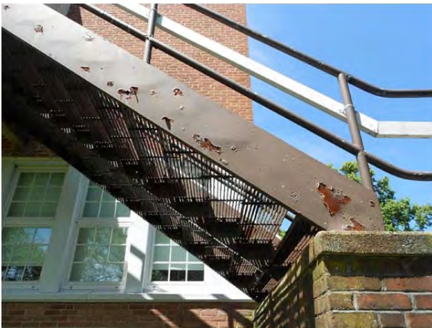
Gymnasium egress stair stringers have rusted completely through and in danger of failure.
