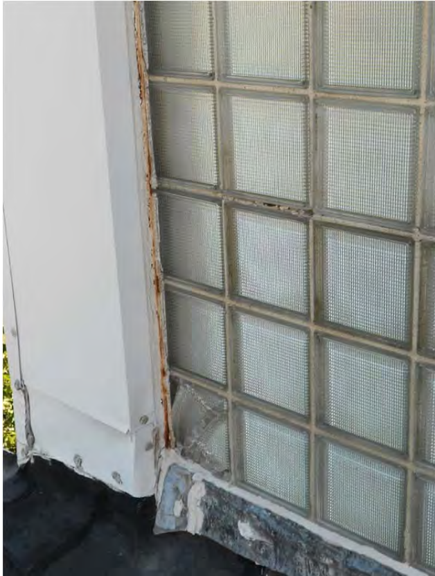
Failed glass block wall through crumbling mortar joints, rusting reinforcing, and shattered glass units
