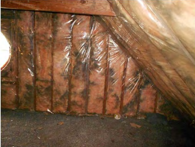
B wing's attic, while well insulated, is heavily compromised by moisture and possible mold.
