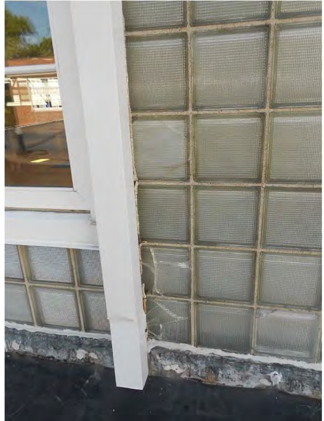
Water intrusion is possible through failed sealant joints at aluminum panning
