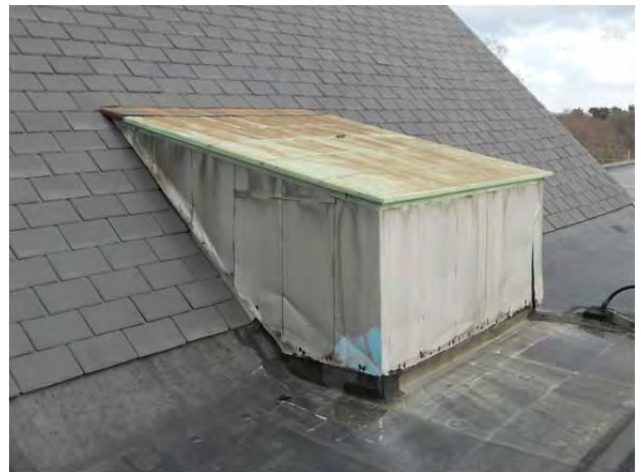
Shed at south side of original building houses HVAC equipment
