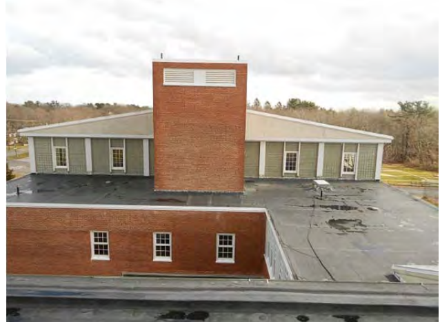
A wing membrane roof showing low pitch and ponding
