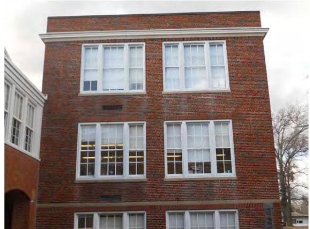
Thin metal thru-wall louvers for unit ventilators are not stormproof and could allow water infiltration.
