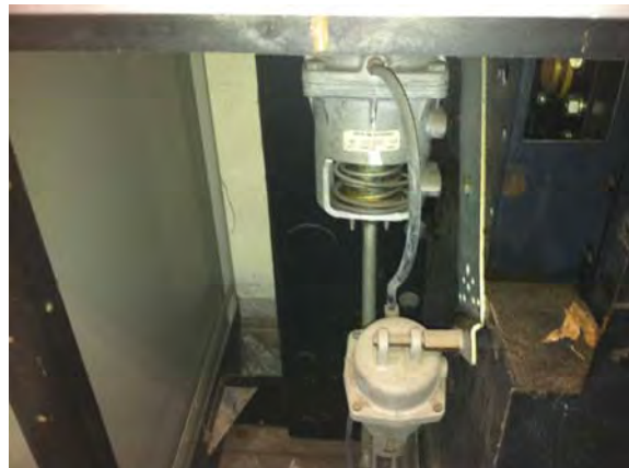
Unit ventilator pneumatic controls (unit interior)
