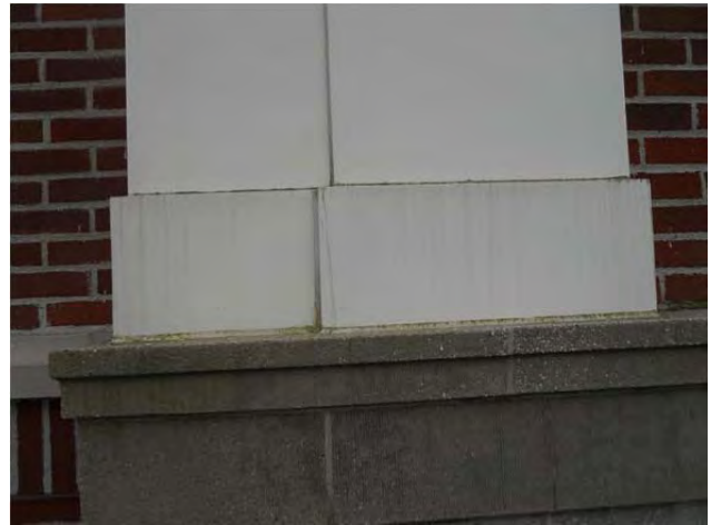
Sealant joints at GFRP pilasters with vegetation and staining.
