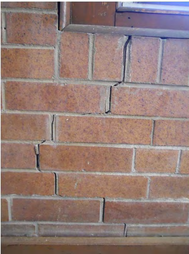
Crack above the door head, west elevation of the southwest stair in B wing.
