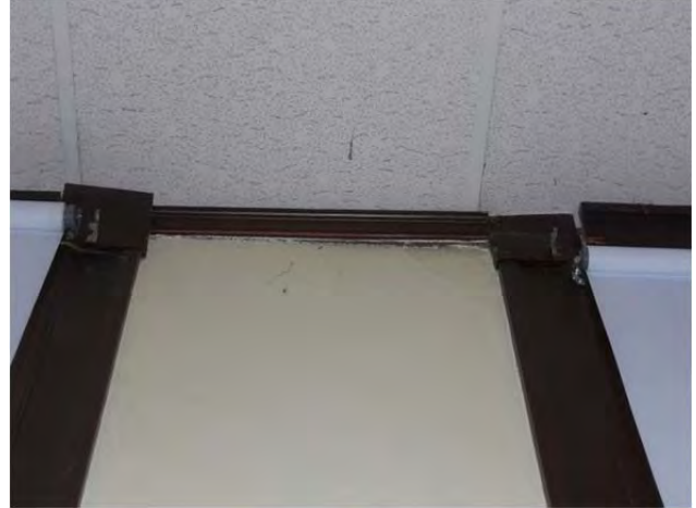
Wood window trim in B wing with water damage
