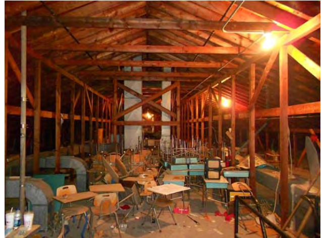
The expansive attic over the A wing classrooms is used for storage and mechanical.
