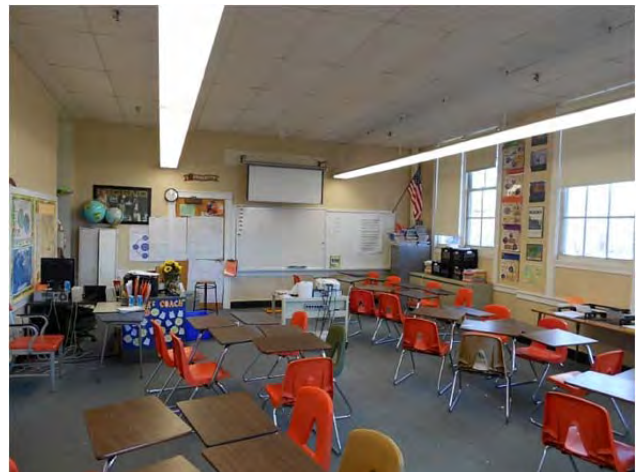
Original plaster ceilings in B wing are covered with suspended acoustic tile ceilings.
