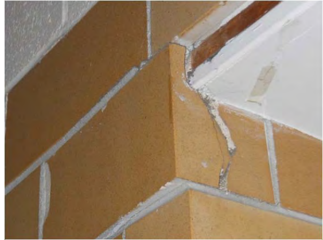
Cracking of the glazed block walls in A wing
