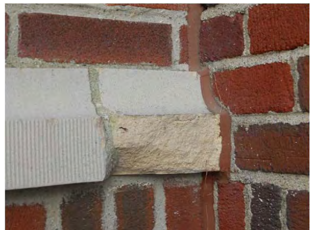
Broken piece of terracotta stone on B wing.
