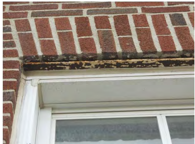
Corroded steel lintels at B wing require cleaning and repainting.
