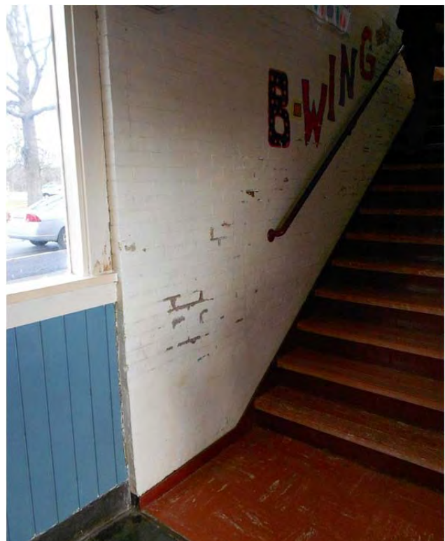
Painted exterior masonry surfaces throughout the building typically have peeling paint.
