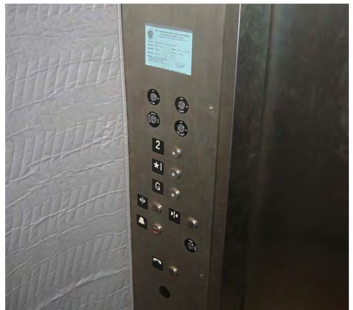
Elevator controls are compliant
