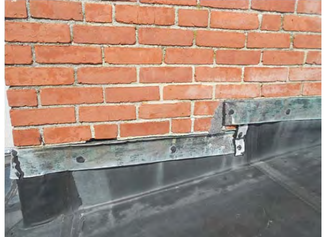
Bent flashing @ mechanical gym mechanical
