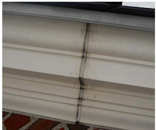
Large sealant joint at butt seam of GFRP raking eave
