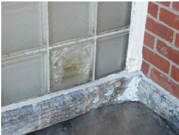
Exterior face of glass block shattered from freeze-thaw exposure.
