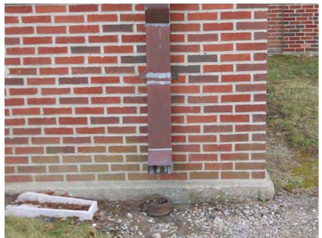
Downspout at B wing with no connection to an underground system or splash block
