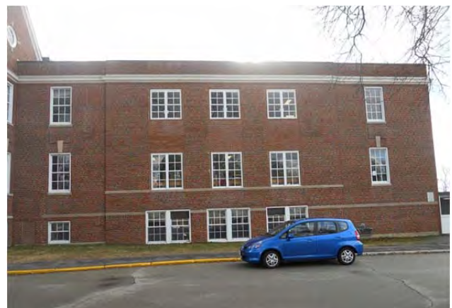
North elevation of B wing with the center bay modified where original spandrel windows were removed
