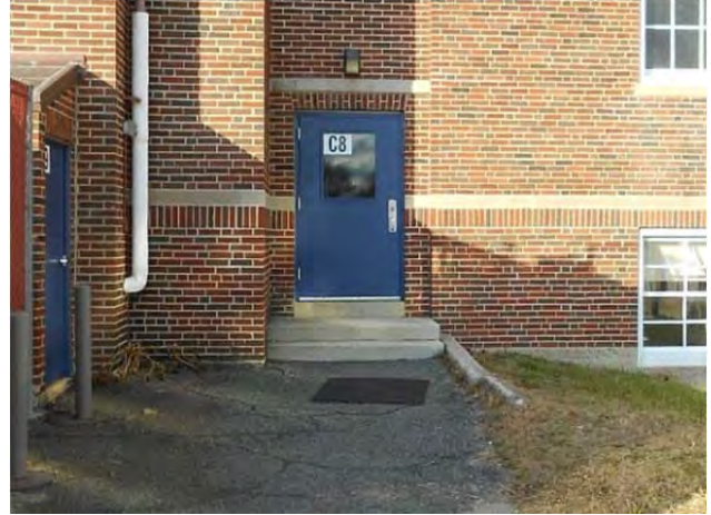
Some exterior stairs have no guard or hand rails.
