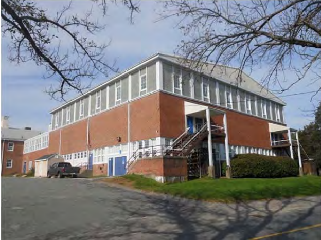
Gymnasium exterior egress stairs are beyond repair
