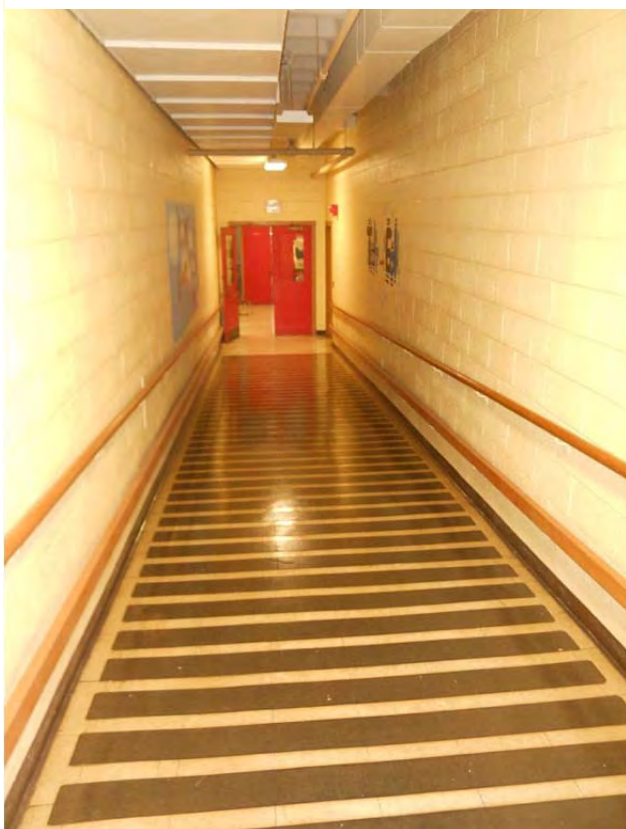
Many ramps are missing one or both required landings
