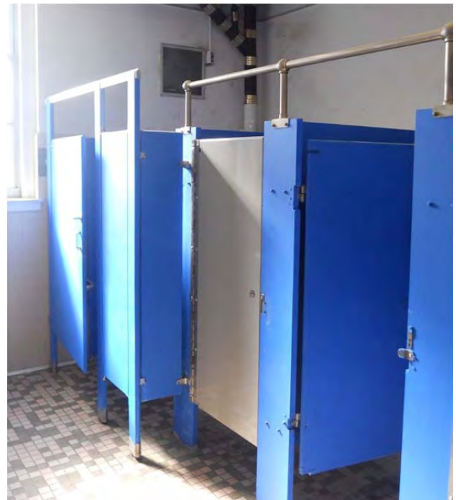
Modified restrooms are not in good condition and need to be renovated in their entirety.
