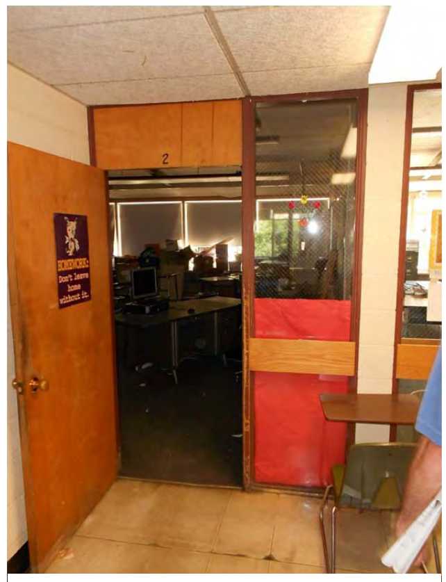
C wing doors, frames, and glass are antiquated
