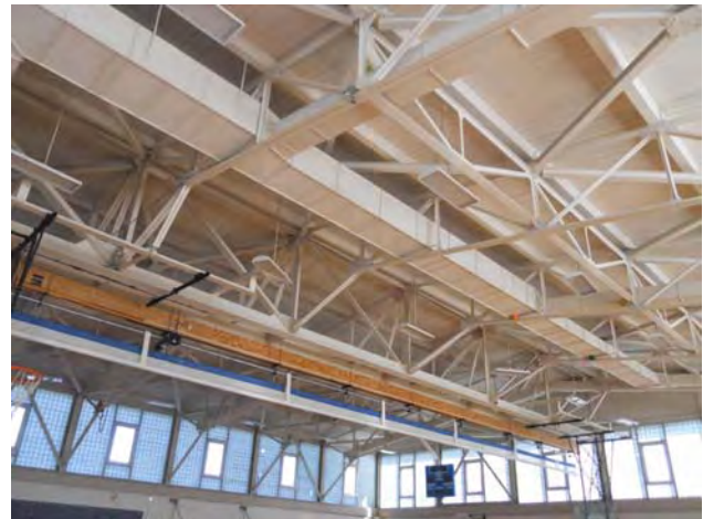
Structural wood decking, wood purlins, and clear span steel roof structure at gymnasium roof.
