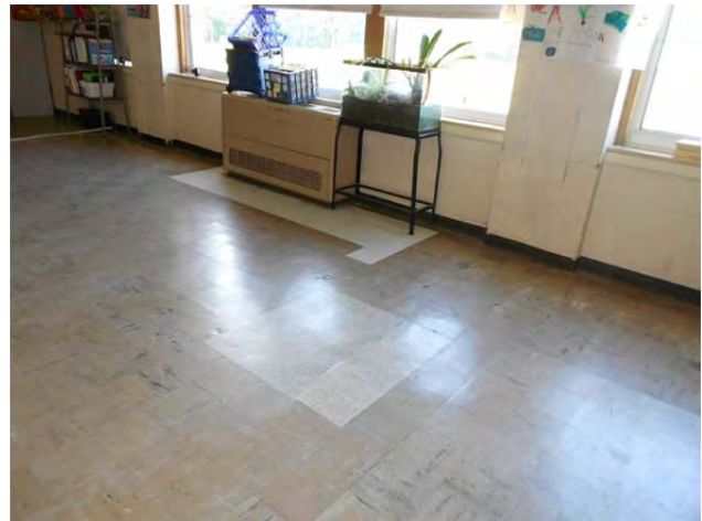
Patched vinyl tile floors are present in all wings
