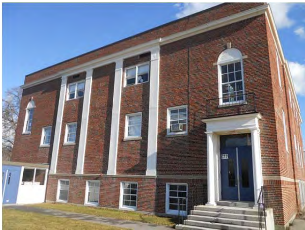
West elevation of B wing heavily modified with non-original windows
