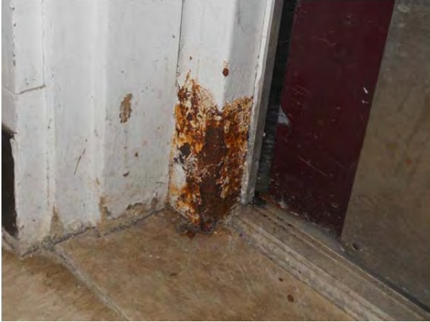
Rusted metal frames are typical conditions at all exterior doors
