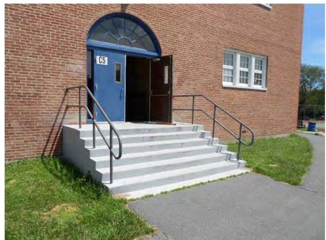
Egress stairs are close to compliant. This stair in A wing only lacks compliant guardrails.
