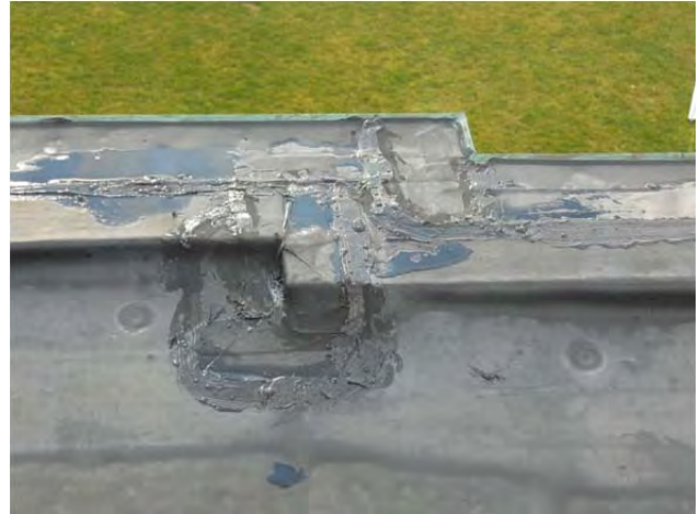
Coping at the flat roof with EPDM seam on top of metal coping and demonstrating past maintenance
