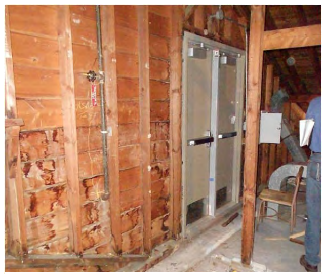
New roof access doors in A wing's attic. Note the old water staining to the left.
