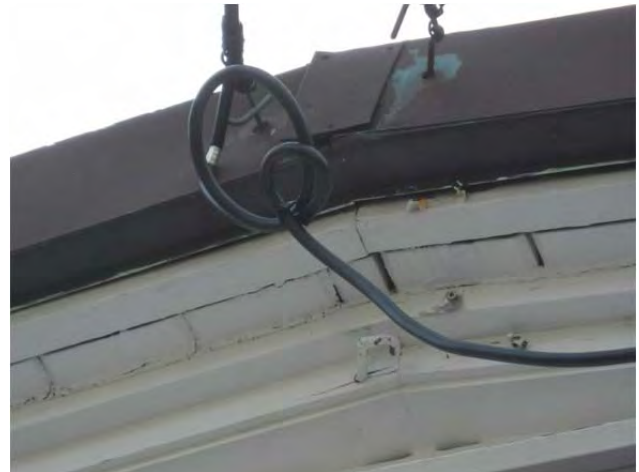
Exposed structural deck at the gable end of C wing is showing signs of exposure to moisture
