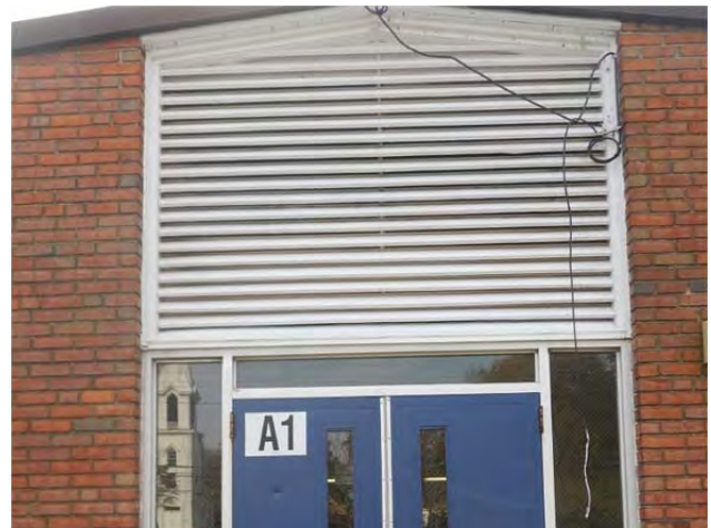
Wood louvers are straight bladed with no provisions to stop water infiltration.
