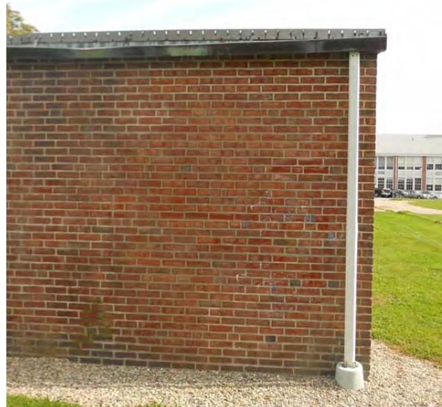
C wing gutters, where they exist at all, have been damaged by ice and snow
