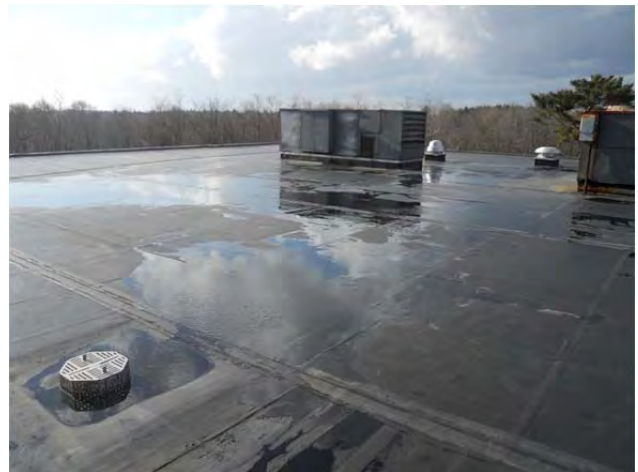
Ponding of water on the EPDM roof on B wing
