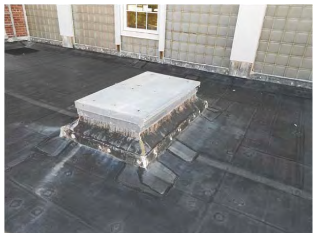
Failing roof curb and hatch adjacent to gym
