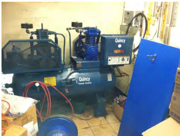
Air Compressor serving school pneumatic controls
