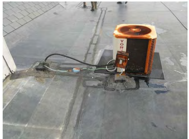
Corroded roof top equipment beyond its useful life
